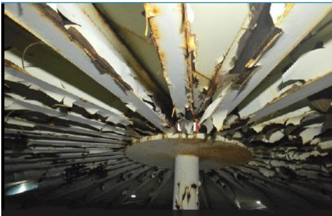
Exbourne (W) – Close up of coating failure on ceiling.
