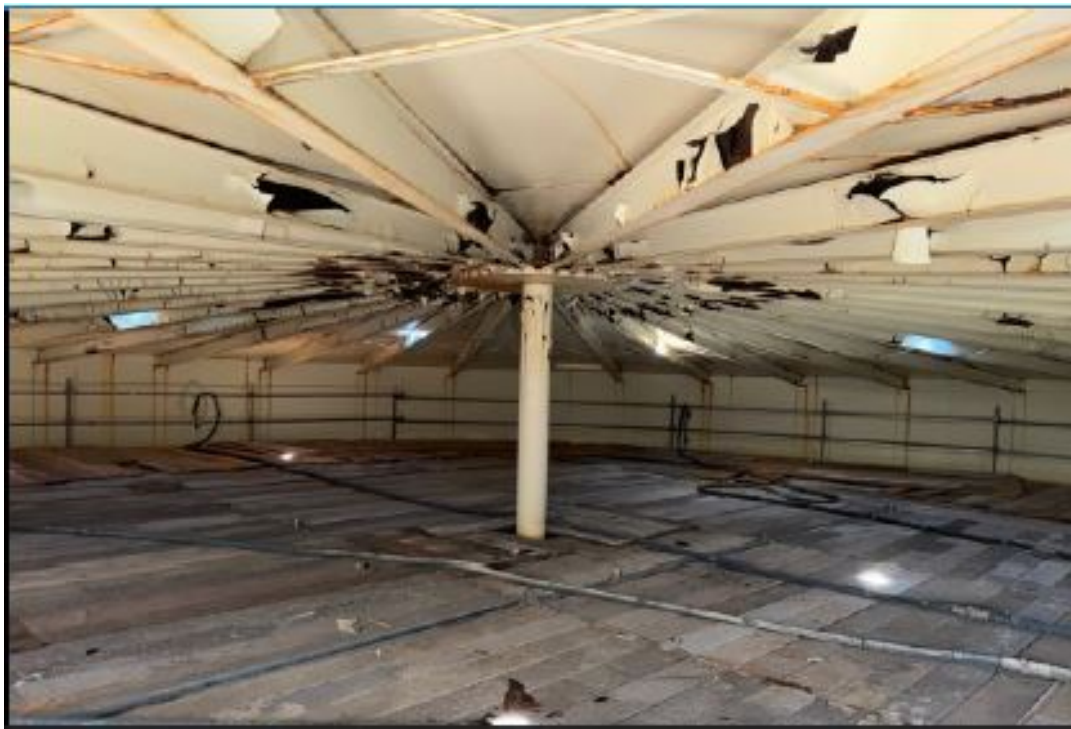
Exbourne (W) – View of interior ceiling and coating failures.
