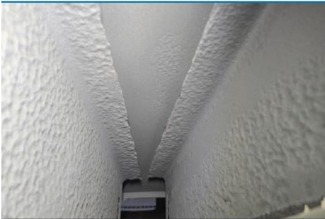
Exbourne (W) – Post-sandblasting of rafters showing pitting.
